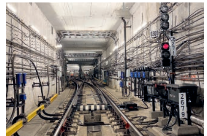
The wayside equipment of the signaling systems in the Moscow Metro
