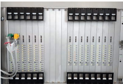
RUVIO relay controllers of HIS-EL in the Moscow Metro Solntsevo electric depo
