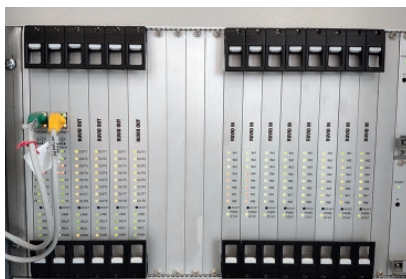
RUVIO relay controllers of RCBI-EL in the Moscow Metro Solntsevo electric depo
