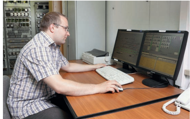
Service engineer checks the operation of a CBI-E system installed on the Moscow Railway
