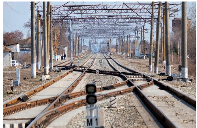
In May 2025, the Signaling Division of GC NPS implemented a CBI system at the Müsüslü station (Azerbaijan)
