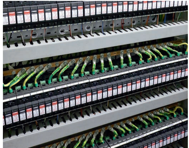
The surge overvoltage and input protection device
