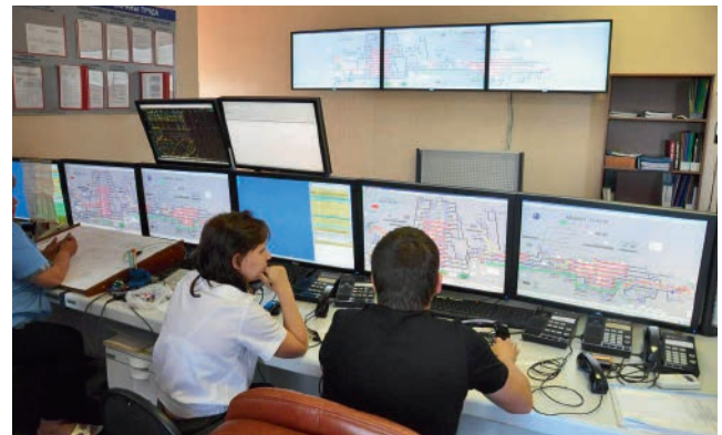
Local Control and Supervisory System (LCSS) in the RBI-E hybrid Interlocking system
